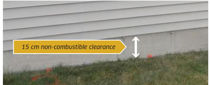
HAZARD FACTOR 7: GROUND TO SIDING CLEARANCE
