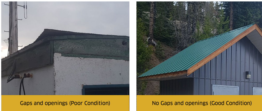
Figure 1. Example of class A rated (metal) roof in poor conditions with gaps and openings that allow ember penetration (left) and good condition (right), with no gaps or openings.
