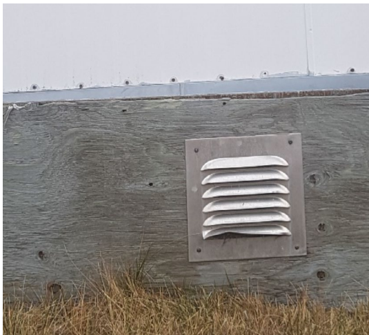
15 cm non-combustible clearing absent
