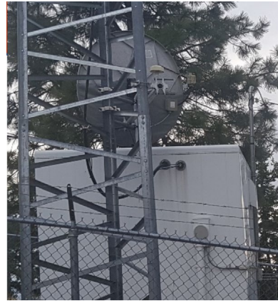
Figure 5. Example of critical infrastructure components that can be damaged by ember accumulation
