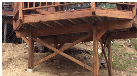
Deck with non-combustible surface and no combustibles stored below
