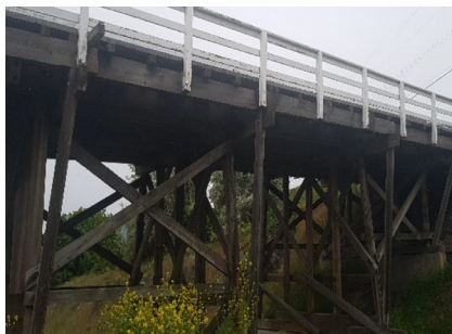
Figure 6. Example of bridge construction gaps and cracks where embers can penetrate and lodge
