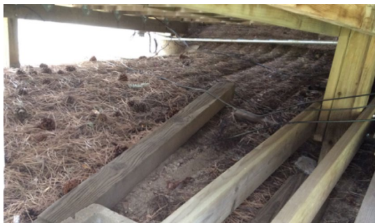
Open foundation with combustible debris
